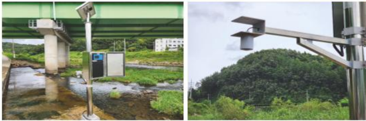
Flood prone road (Sejong City)
